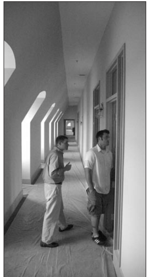
Above Left: Mr. Carey, Mr. Lassiter, and Mr. Heubeck explore the large classroom that has replaced the history offices on the 2nd floor of Carey Hall Above Right: Mr. Hastings and Mr. Lauer examine classrooms from the Carey Hall's new 3rd floor corridor
